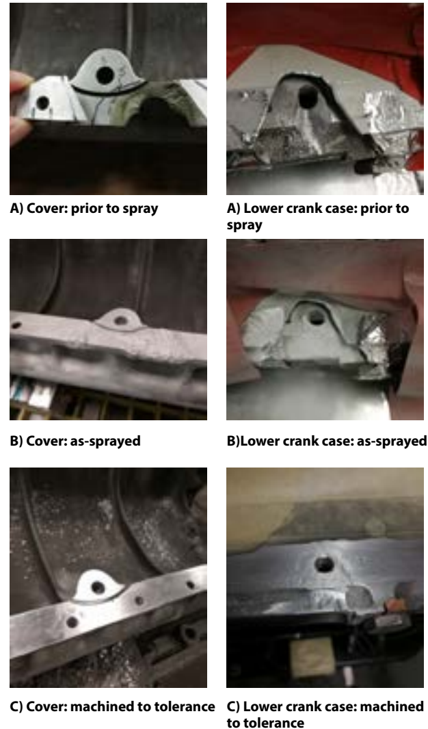
Figure 6. Gipsy DH Major 10MK1-3A engine top cover and lower crank case flange repair by cold spray.
